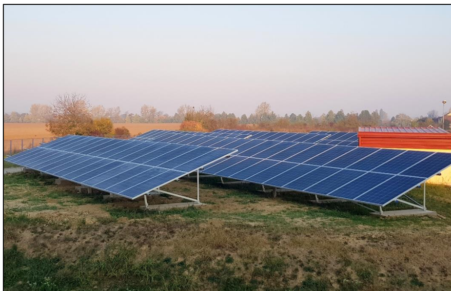
Figure 10. 380kW photovoltaic power plant
